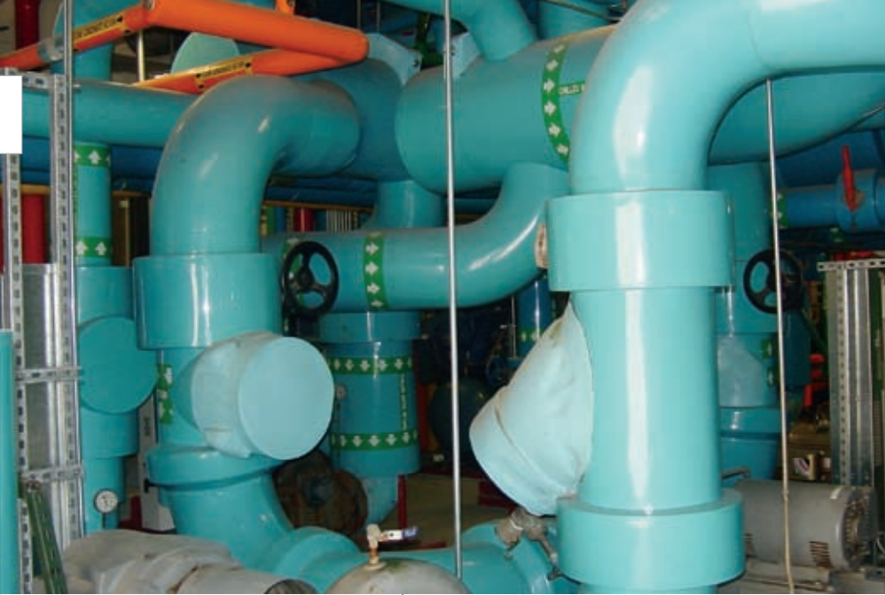
Typical chilled water piping that was replaced in the central plant at Methodist Charlton Hospital in Dallas.
